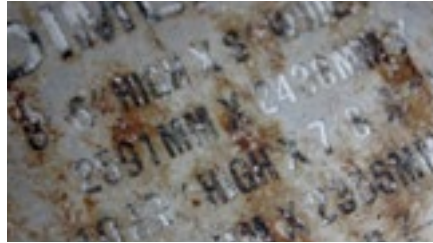
Road Salt Corrosion Damage
